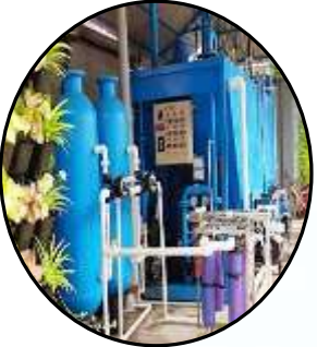
WTP/RO/STP Plant Maintenance
